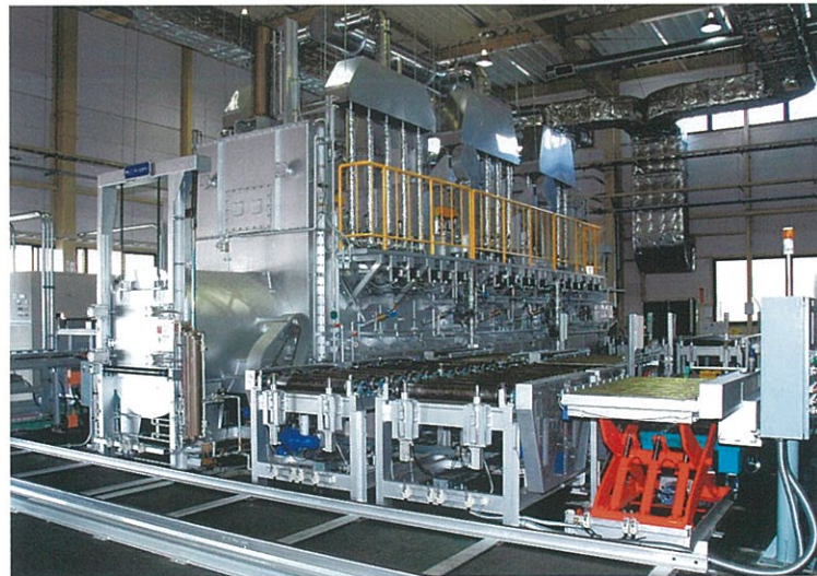
連続式無酸化焼鈍炉 Continuous type non-oxidation annealing furnace
